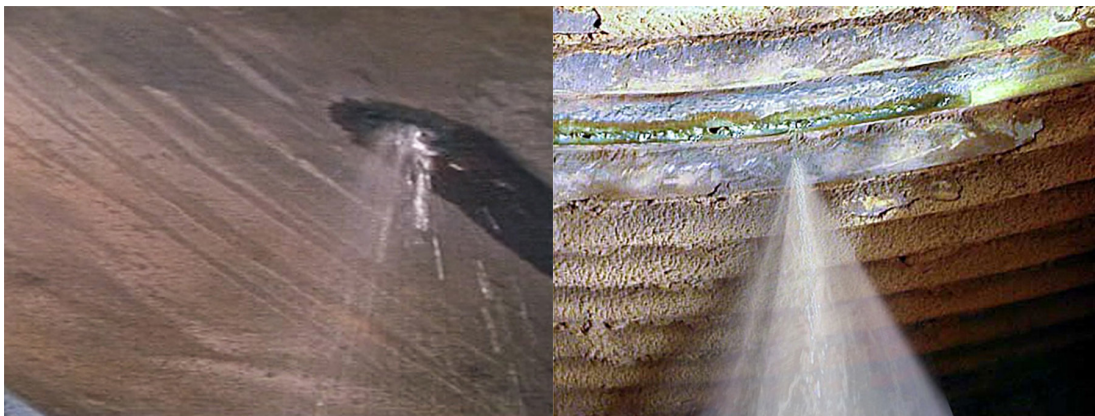
Leak in a non-pressurized spray cooling system (left) vs. leak in a pressurized tubular system (5 gal/hr vs. 16,000 gal/hr)
