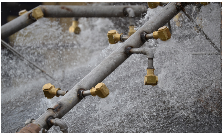
Spray bars in a non-pressurized spray cooling system
