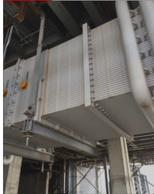
Supported Duct Work
