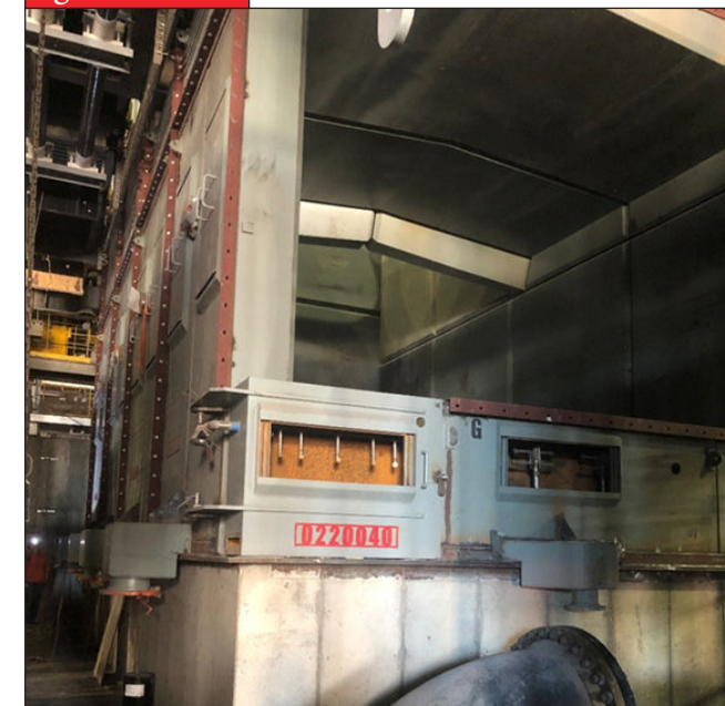
Systems Spray-Cooled Drop Out Chamber, Showing the Interior Walls
