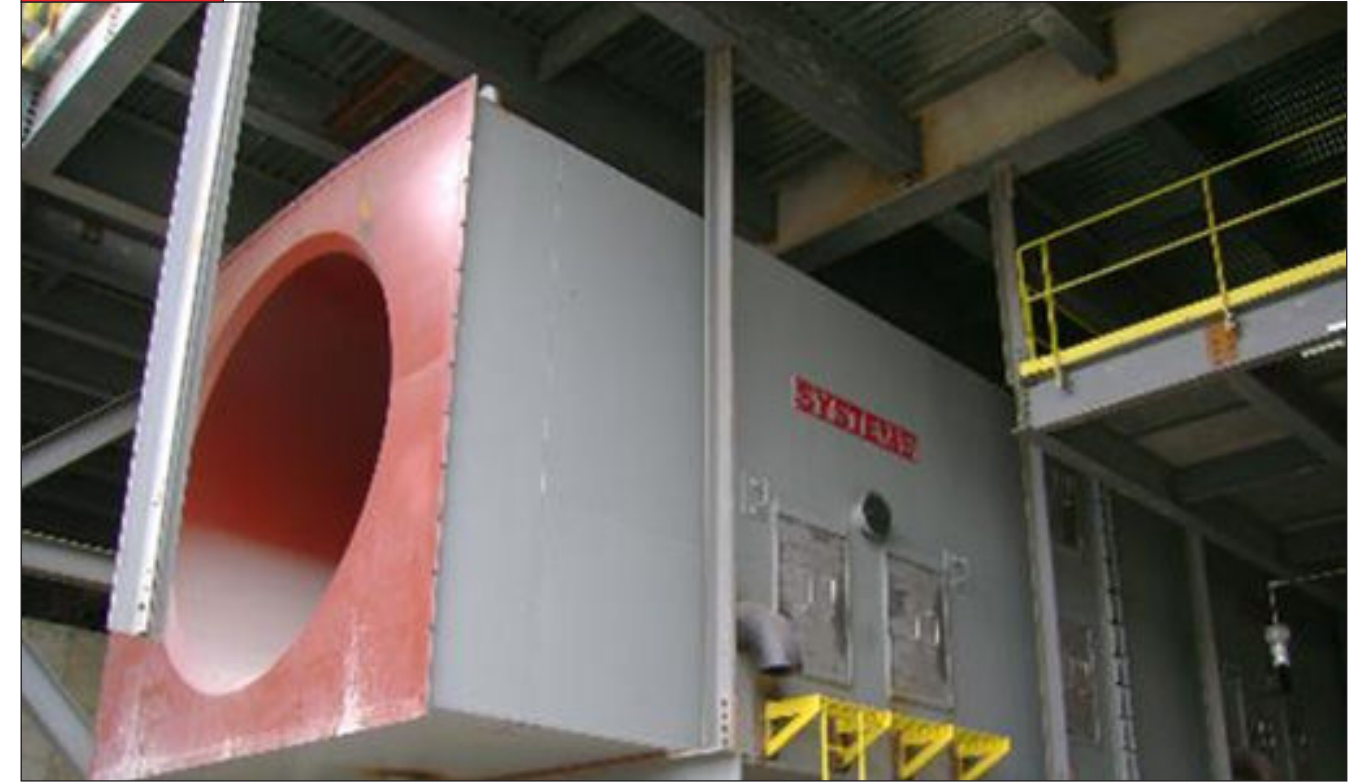
Systems Spray-Cooled Ductwork
