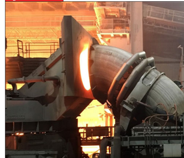
A Systems Spray Cooled Fixed Elbow (left) Mating With a Movable Tubular Elbow (right) and a Tubular Vertical Downcomer Duct.
